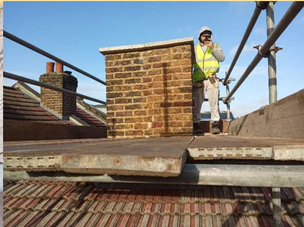
HEET arranged for what remained of the chimney stack to be taken down. Removing the risk of structural collapse.
