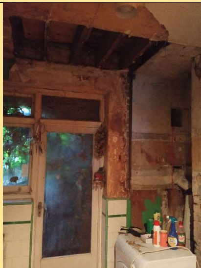
Toilet leak needed fixing to prevent further deterioration to house
