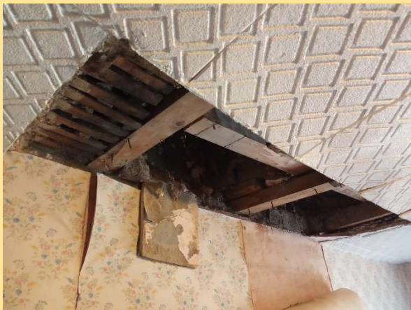
Bedroom ceiling where chimney stack had been incorrectly supported
